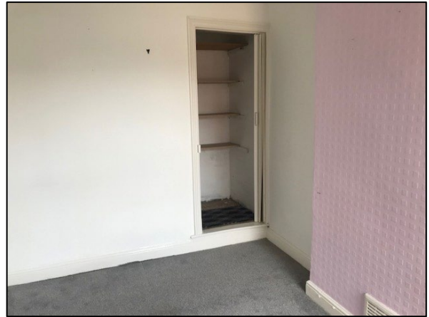
Photograph showing the second of the first floor bedrooms which will remain.
